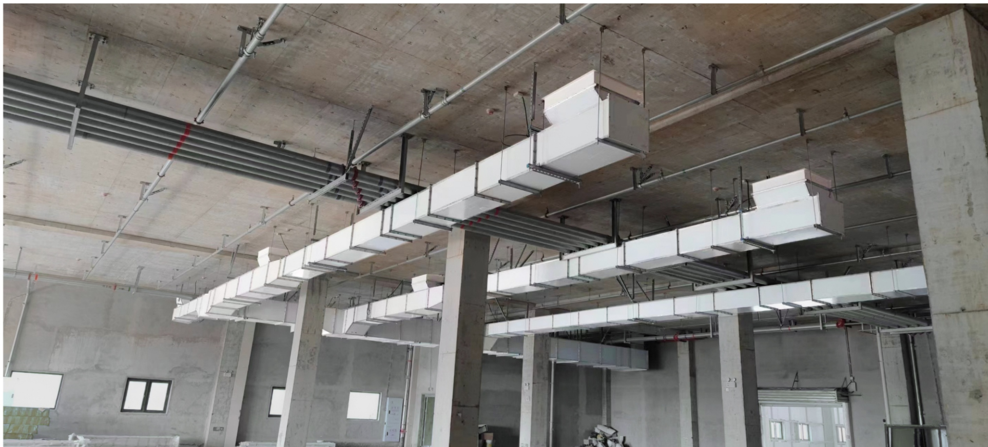
现场实际安装图 field installation
